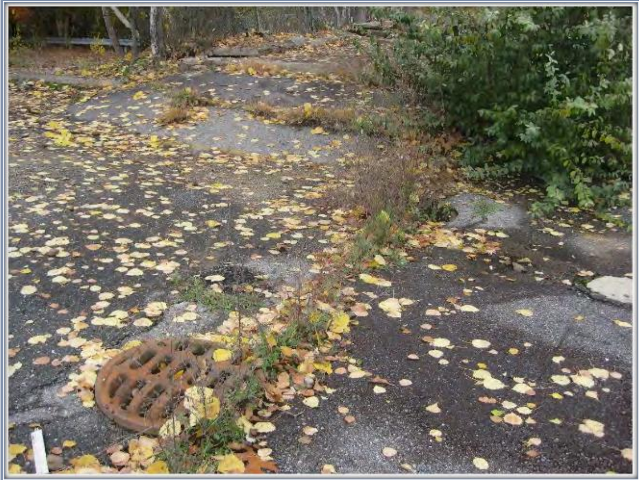
Photo 4: Uncovered manhole near Components Laboratory Building, 2018
