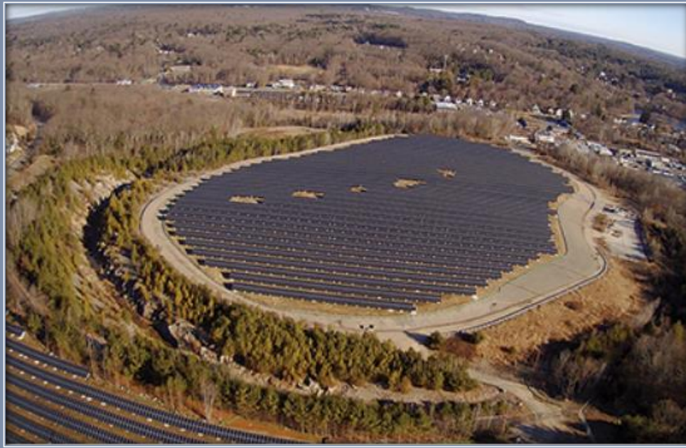
This photo captioned, “50 MBTA Access Road – Ashland, MA,” originally appeared in the article, “Aldon Electric completes 5.8MW Ashland, Mass. solar landfill project” (2020, April 17) in New England Real Estate Journal . https://nerej.com/aldon-electric-completes-5-8mw-ashland-mass-solar-landfill-project
