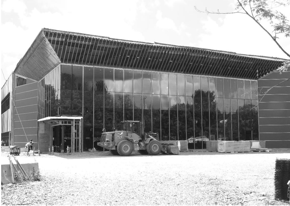
Second biotech building under construction at Bedford Woods Office Park, off Middlesex Turnpike
