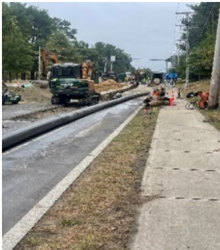
Crosby Drive Sewer Force Main
