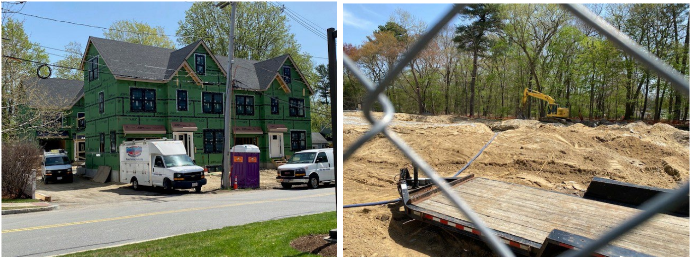
Construction underway on multifamily housing projects at Webber Ave (left) and Loomis Street (right)
