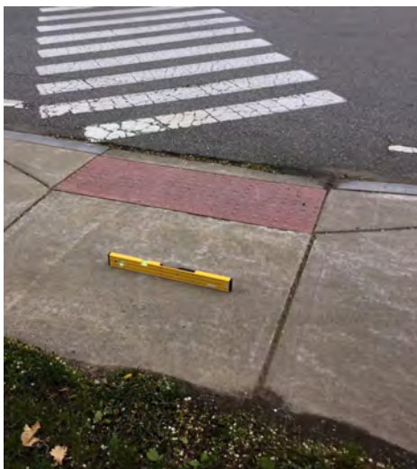
South Rd. @ Railroad Ave. Well constructed AAB compliant ramp with slight threshold lip maintenance issue
