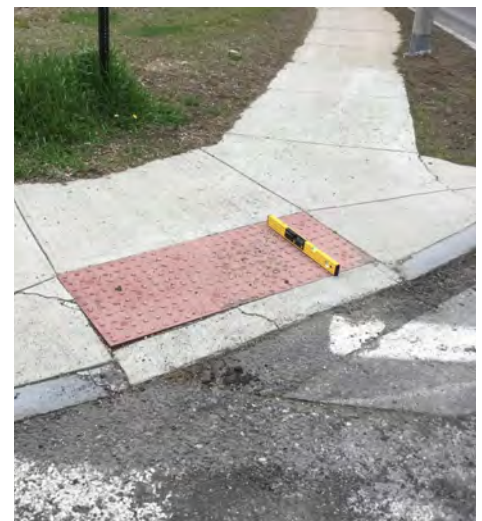
The Great Rd. @ Walsh Rd. Recently Constructed AAB Compliant ramp, prematurely cracking/tactile panel lifting
